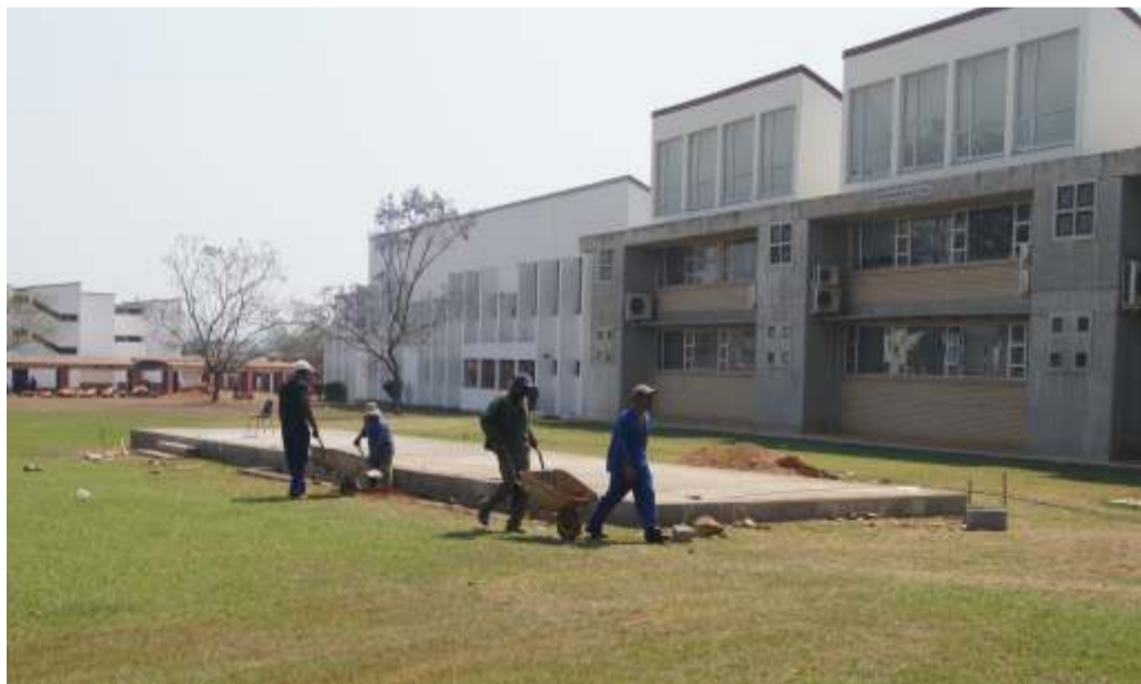
A permanent stage under construction next to the Engineering building at Kwaluseni campus (Pic by Tengetile Mpila)
